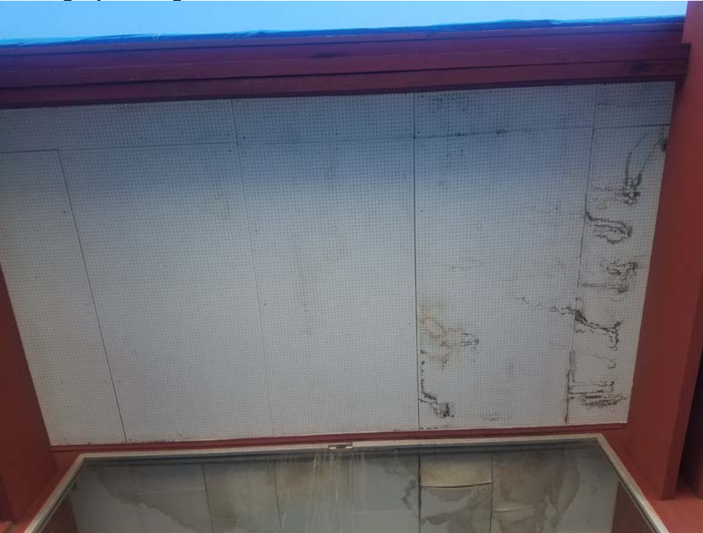
HM-05: Exterior Eaves, Transite® Asbestos Paneling, 15% Chrysotile.
