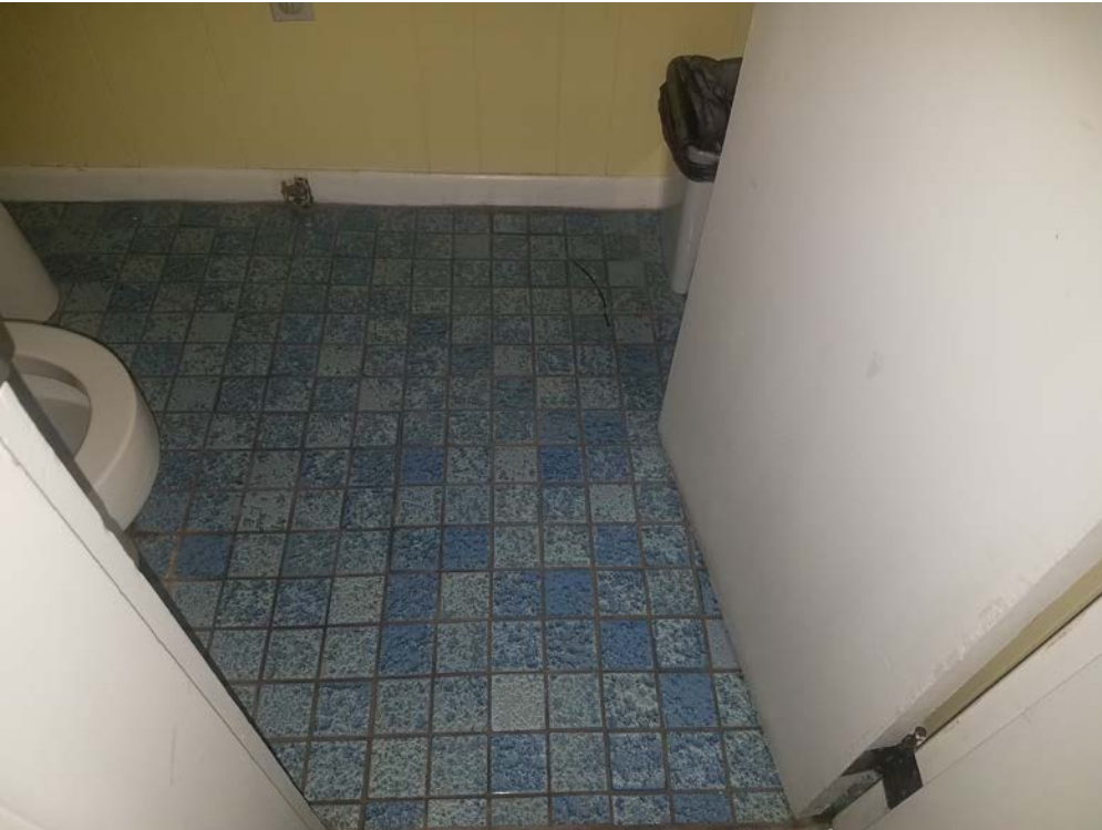
Ceramic Tile applied to concrete in the Bathroom. Not a suspect ACM.
