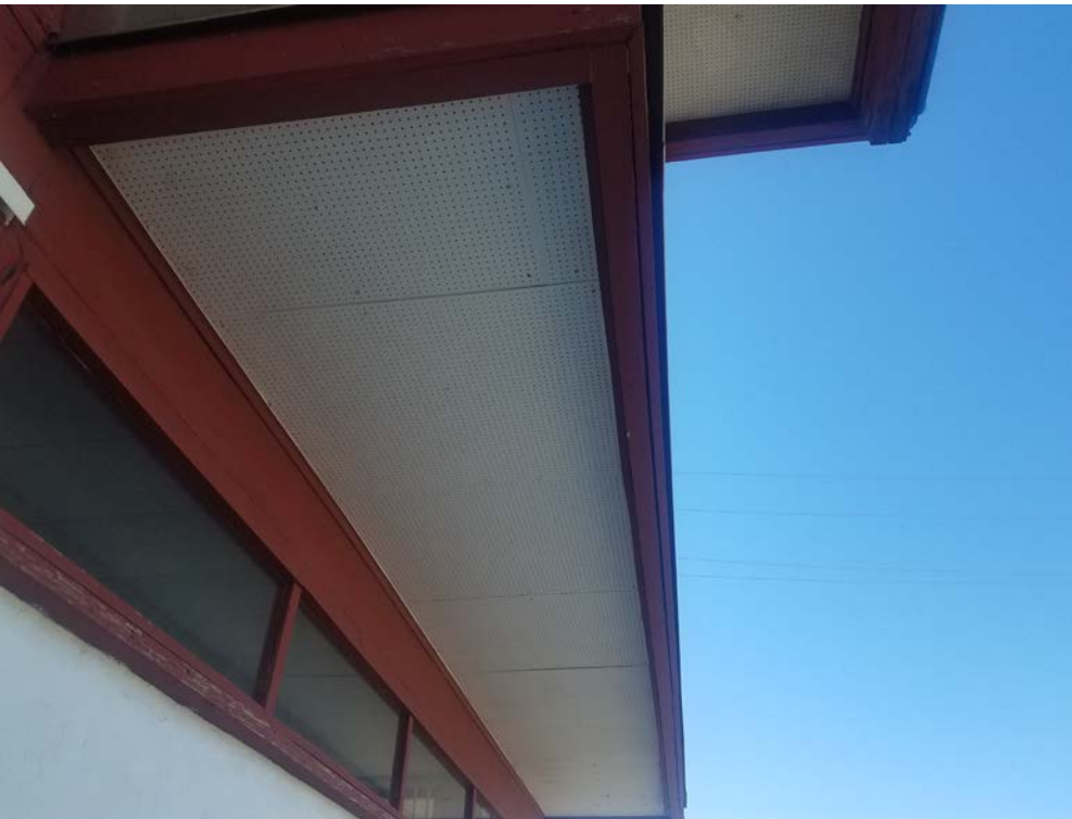
HM-05: Transite® Asbestos Paneling. See paneling applied to upper roof also.
